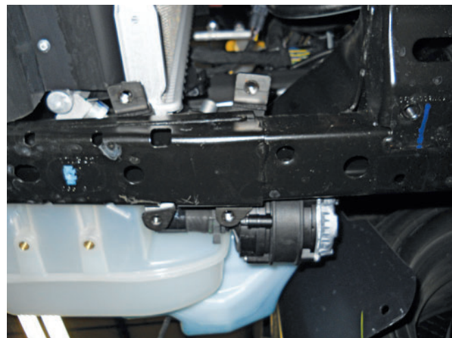
4. Place the intercooler pump mounting bracket (1318-8C4191) (lower) in position under the upper brackets and install the six (6) bolts (161821, found in 1318-TVSHWKH) (13 mm socket).
